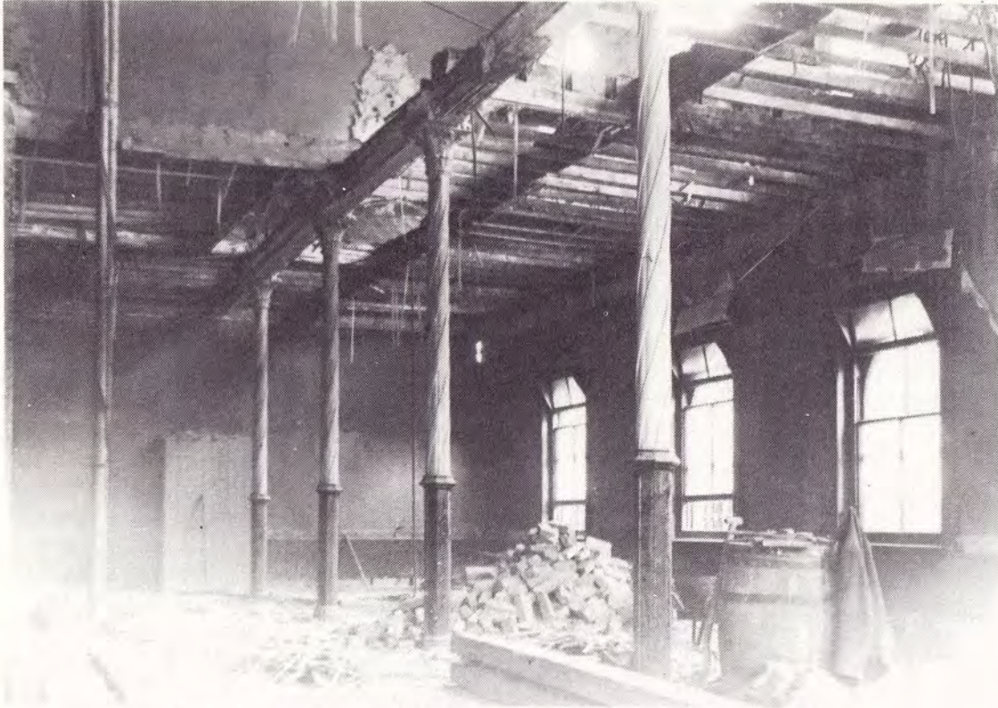
Repairs being undertaken after the floor collapse in 1934. At this date the cast iron pillars in the Council Chamber were removed.
