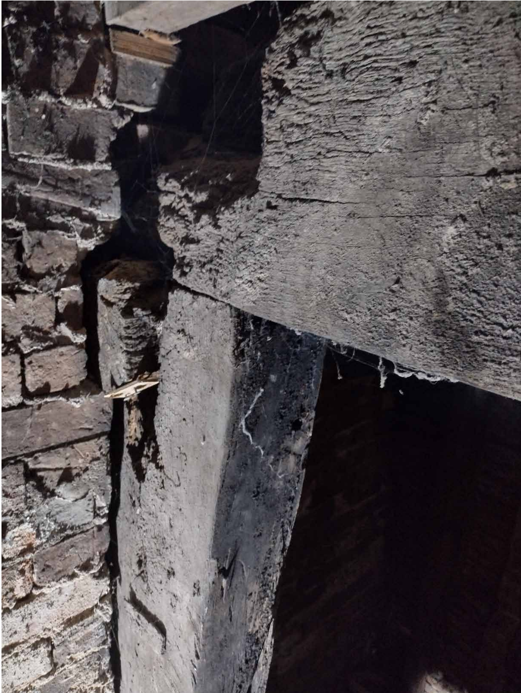
Figure 2: Front range; post and tiebeam at truss 7a, photograph taken from the west [Martin Bridge]
