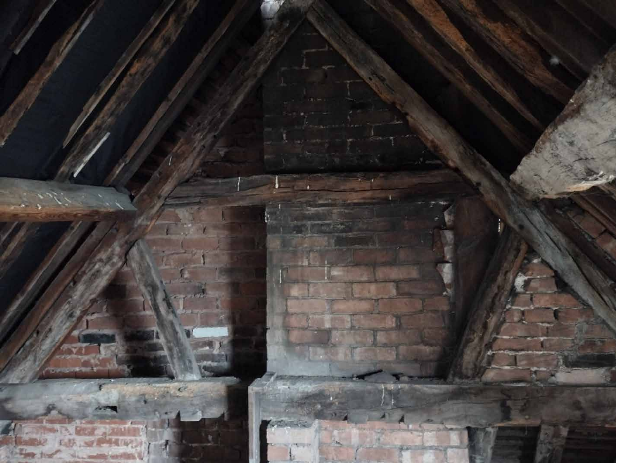
Figure 3: Front range, attic; truss 7b, photograph taken from the east [Martin Bridge]
