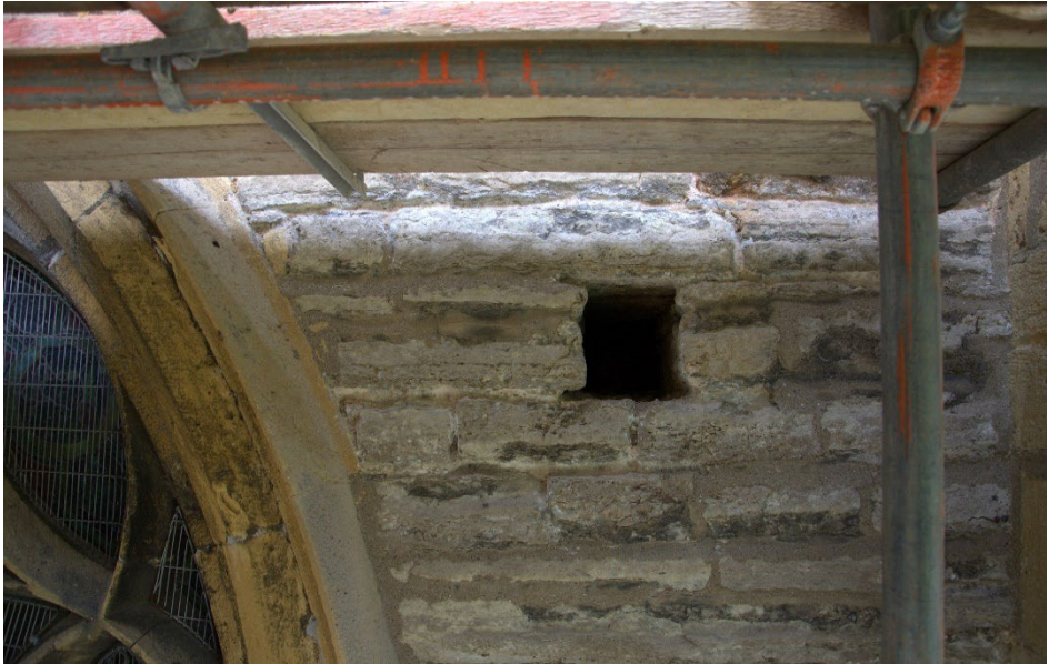
Example of a 'putlog' hole in the masonry, observed with the aid of scaffolding.
